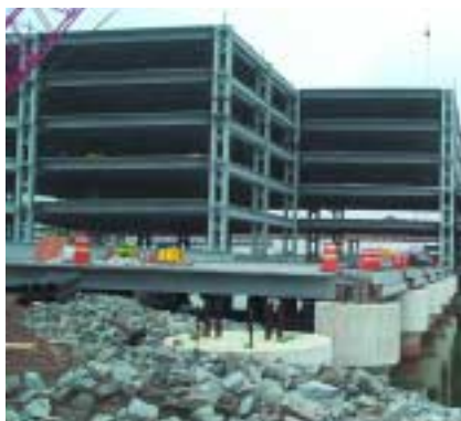
View of construction of the Lot E Garage progressing over the caisson foundations in the drainage waterway.
