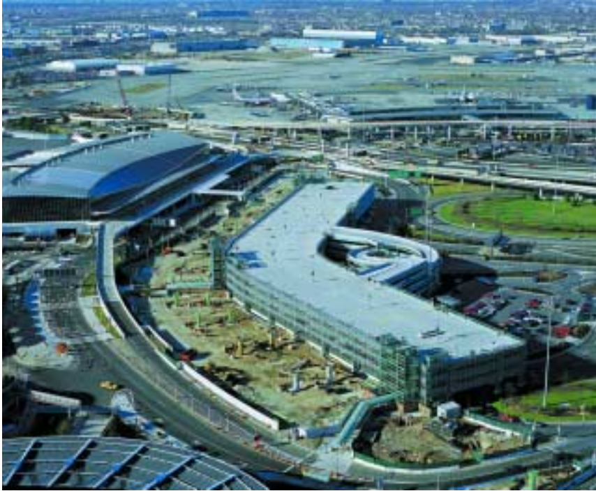
Aerial view of the Green Garage at JFK Prior to AirTrain Construction.
