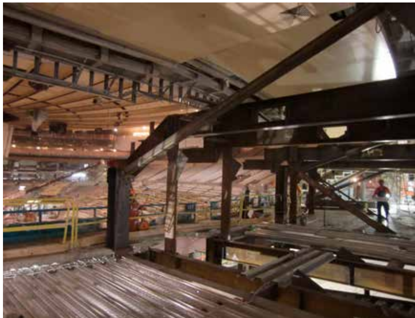
▼ More than 500 pieces of precast seating is supported by more than 50 40-ft-long to 90-ft-long steel raker beams.
